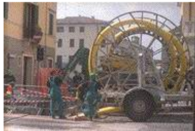
Compact Pipe conveyor
